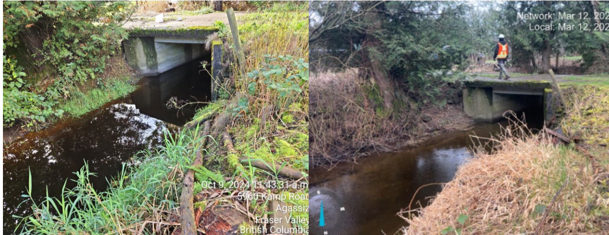
Photo 2.1 Hicks Creek at PDL-A6 in October 2024 (Left) and March 2025 (Right) Looking Upstream at the Existing Bridge
